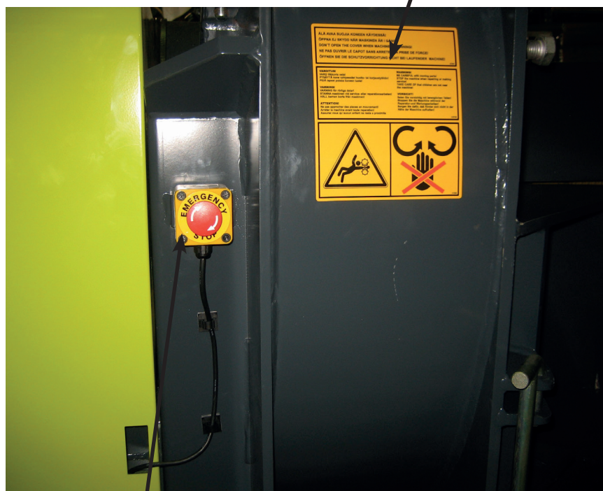
FEEDER EMERGENCY - STOP
